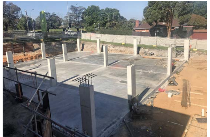
The freshly poured first section of the slab for the ground floor.
