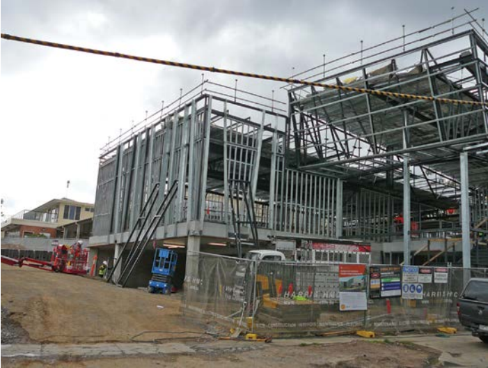
The view of the rear of the building from Warner Avenue - late April...
